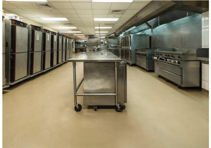
The worn quarry tile in the kitchen and concession areas were replaced with seamless, easy to clean, stain resistant Stonclad
